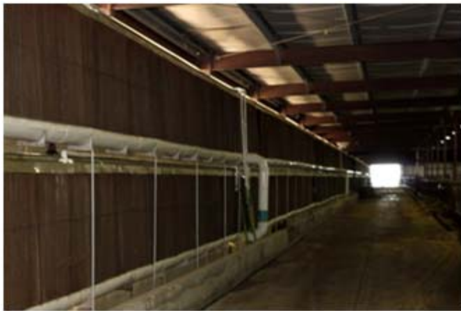
Picture 4. Interior view of the side wall with the air intake made of evaporative panels.
