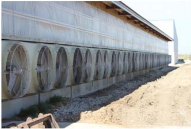
Picture 3. Exterior view of the side wall made up of fans.
