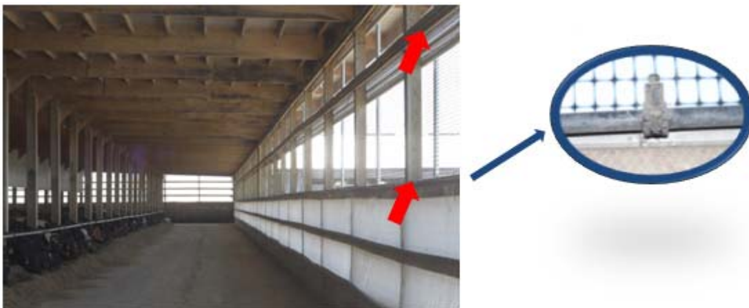
Picture 6. Interior view of the side wall with 2 rows of nozzles (red arrows).
